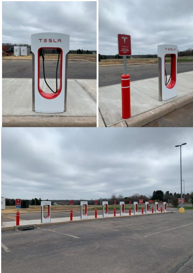
Figure 1: Electric Car charging ports on I 476 in PA. Installed Spring 2021.
